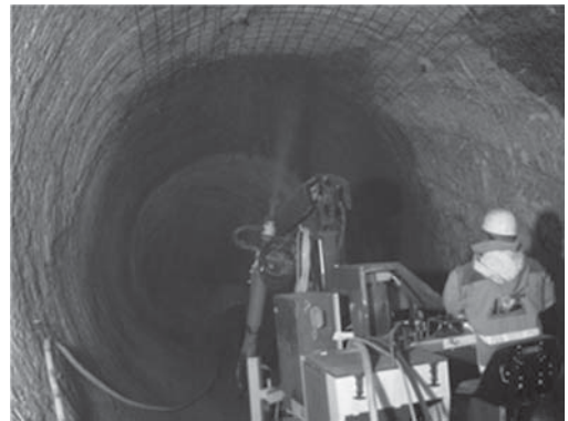
Figure 16. Application of sprayed concrete to the substrate via MEYCO Oruga manipulator prior to the spraying of the membrane (Giswil tunnel).
