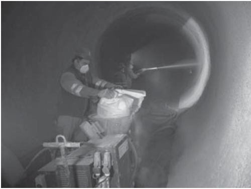
Figure 18. Set-up for the application of Masterseal® 345 with MEYCO® Piccola dry sprayed concrete machine (Giswil tunnel).
