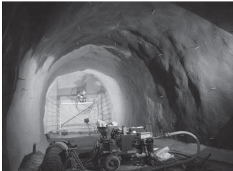
Figure 26. Application of a smoothing layer prior to spraying of the Masterseal® 345 waterproofing membrane (Hirtenberger Ammunition Caverns).
