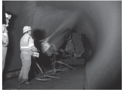
Figure 19. Application of the inner concrete layer with wet-mix sprayed concrete (Giswil tunnel).
