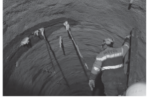
Figure 15. Temporary removal of water seepages before applying the sprayed concrete substrate (Giswil tunnel).
