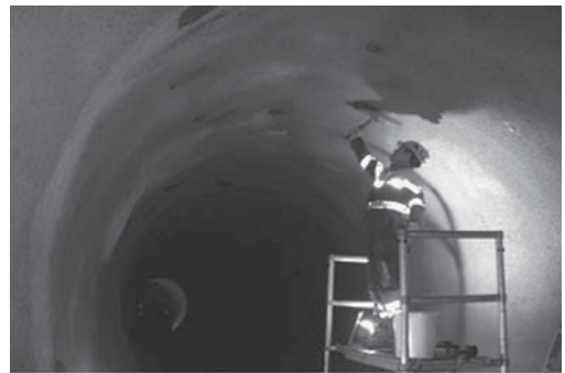
Figure 17. Before the spraying of membrane: removal of the last drip spots through rock bolt holes with injections with MEYCO® MP308 (Giswil tunnel).
