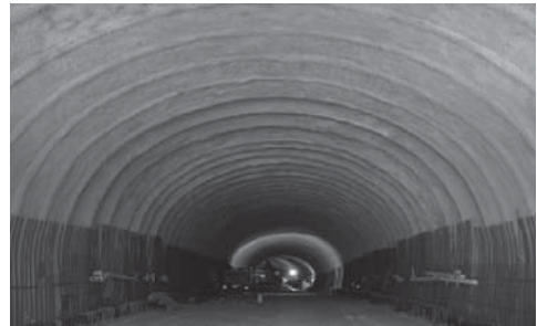
Figure 20. Masterseal® 345 applied to the entire tunnel contour. A final lining of 30 cm sprayed concrete was applied on top of the membrane (Tunnel de Viret).
